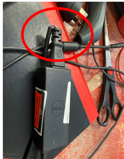
Image 2: Damaged parts at the charger end.
